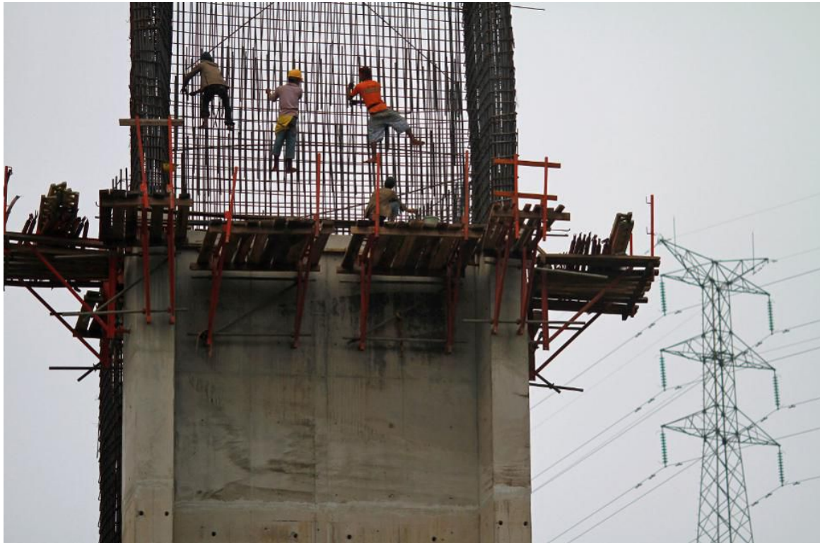
Workers labor on the construction of a highway in Indonesia. (Dimas Ardian/Bloomberg)
